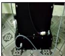
Figure 3: The process of motor wiring system.
